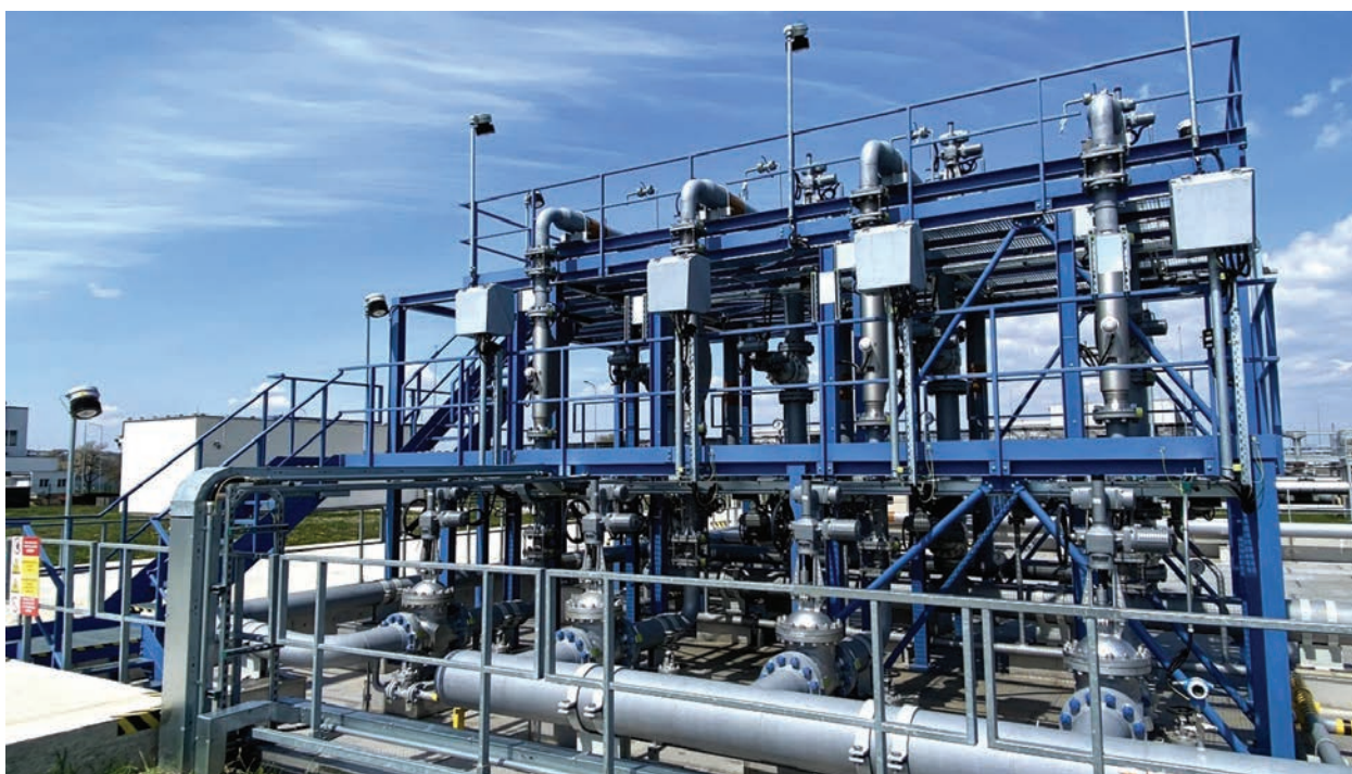
Figure: Oil metering station ADRIA at PS-4 Tupá
