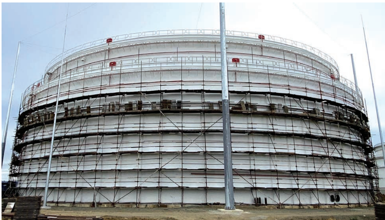
Figure: Crude oil tank No. 236 at PS-1 Budkovce
